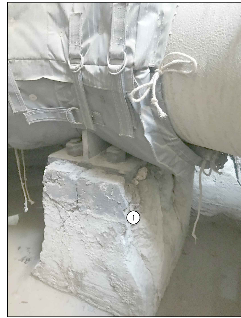
1 SPALLED CONCRETE, SEE REPAIR NOTE 1.
