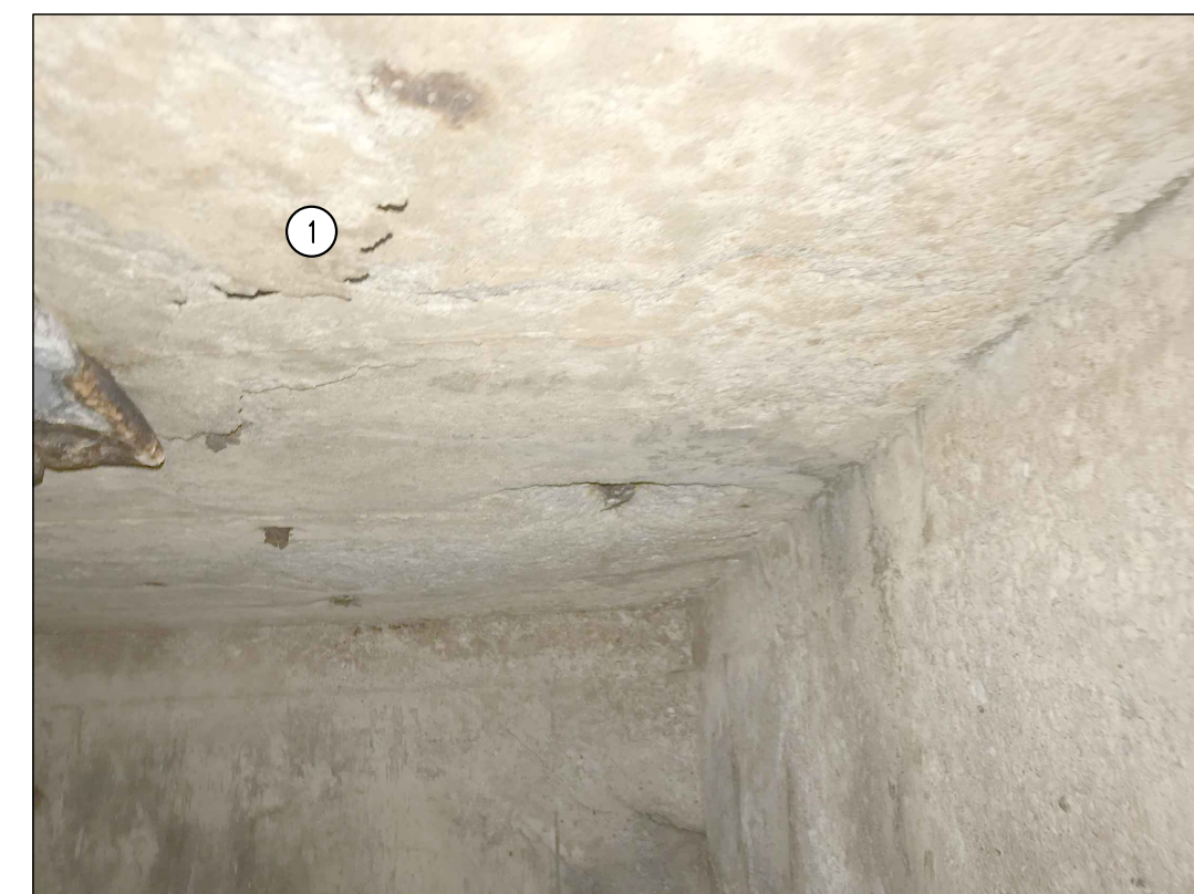
1 SPALLED LID, SEE REPAIR NOTE 1.
