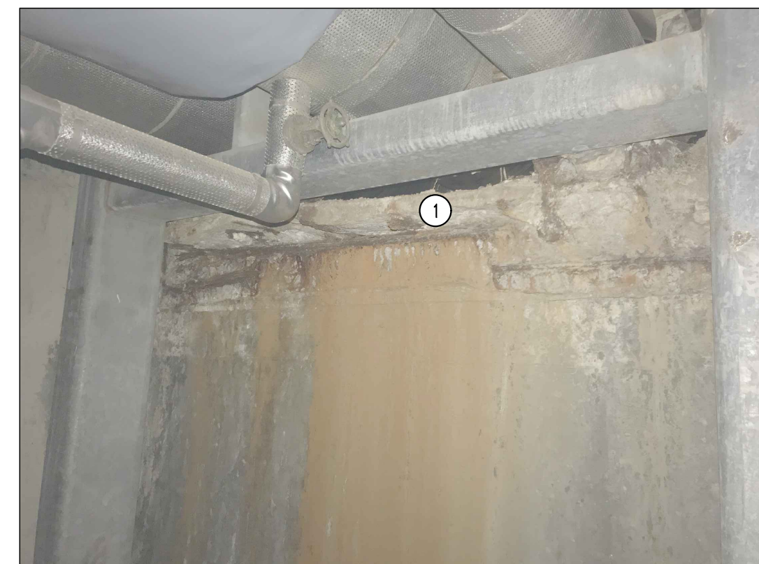
1 SPALLED CONCRETE, SEE REPAIR NOTE 1.
