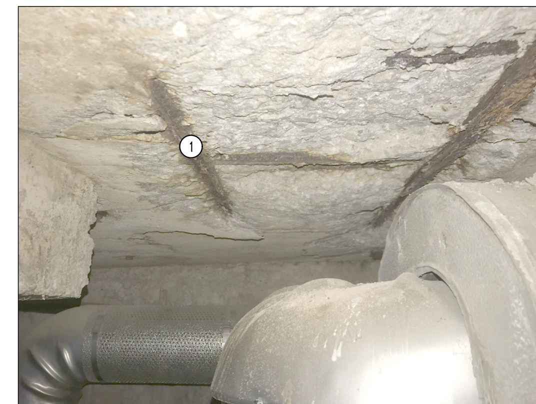
1 EXPOSED REBAR, SEE REPAIR NOTE 3.
