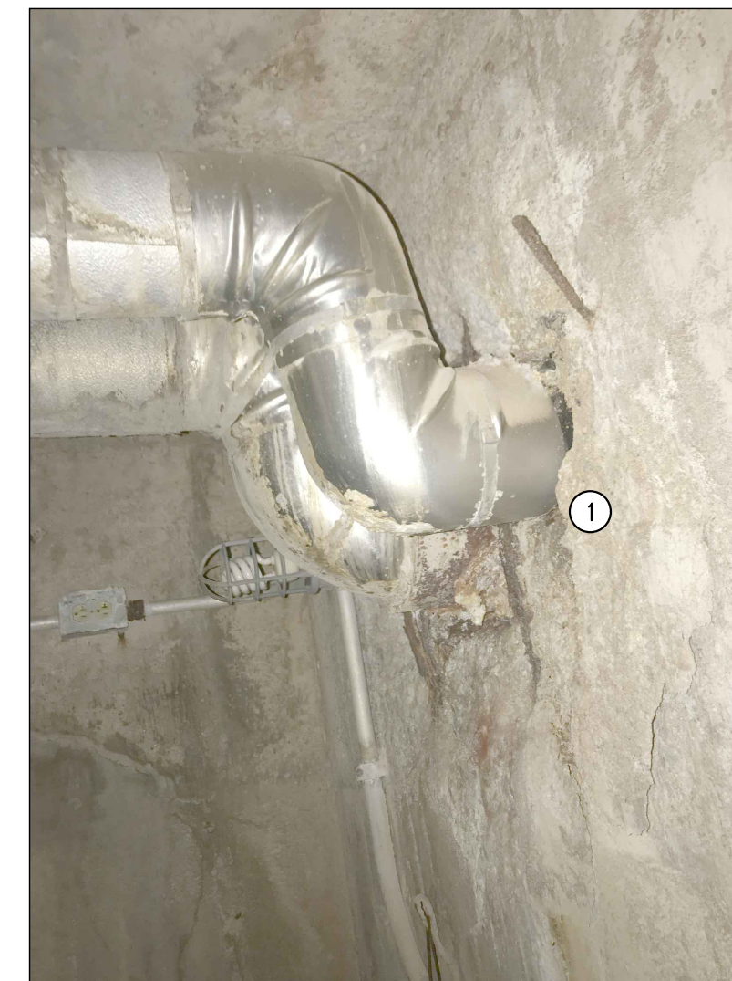
1 SPALLING, SEE REPAIR NOTE 2.
